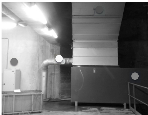
Figure 1. Off-gas ventilation shaft (red dot, yellow dot) with gas sampling pump and sensor cabinet (blue dot) and gas sampling point (purple dot).
